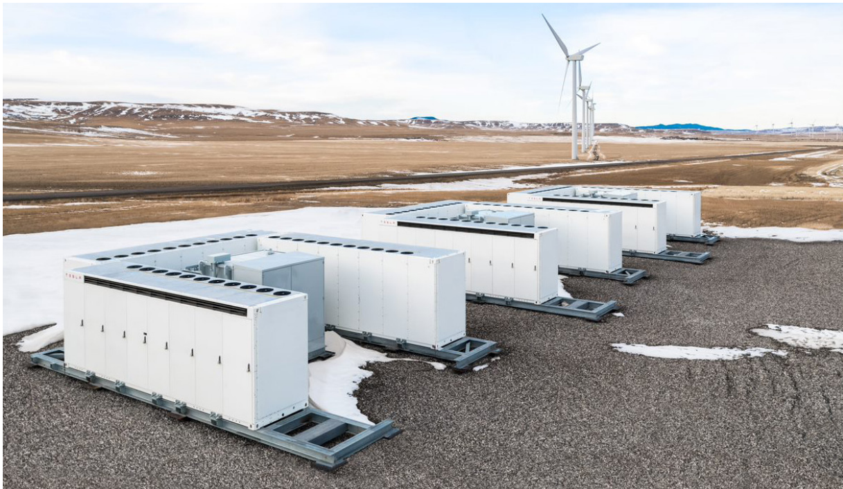
Battery modules located at TransAlta's 10 MW WindCharger facility in southern Alberta - the first utility-scale lithium-ion battery storage facility in Alberta.
